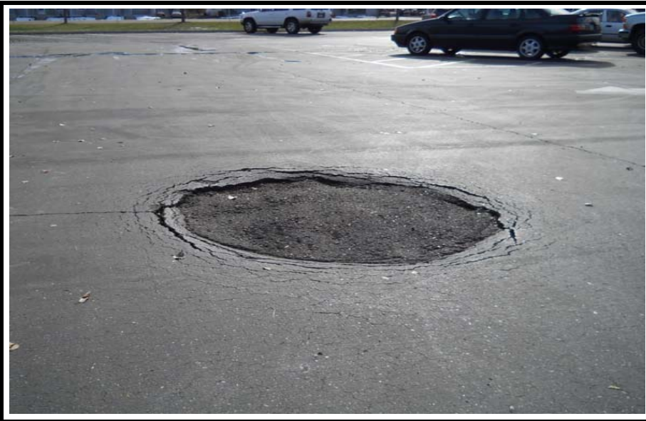
PHOTO NO. 1: Close-up view of major POT-HOLE located within the southeastern student parking area near Boring B-1.
