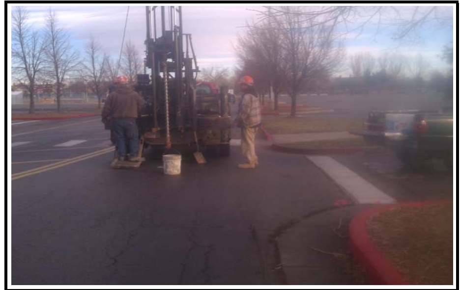
PHOTO NO. 2: View of pavement in general vicinity of Boring No. B-3. Pavement distress/failure adjacent to the concrete curb radius along with longitudinal cracking.
