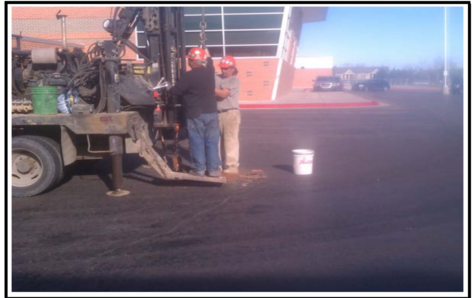
PHOTO NO. 4: View of pavement in general vicinity of Boring No. B-9. Pavement distress of alligator cracking. Note crack sealant applied to increase pavement longevity.
