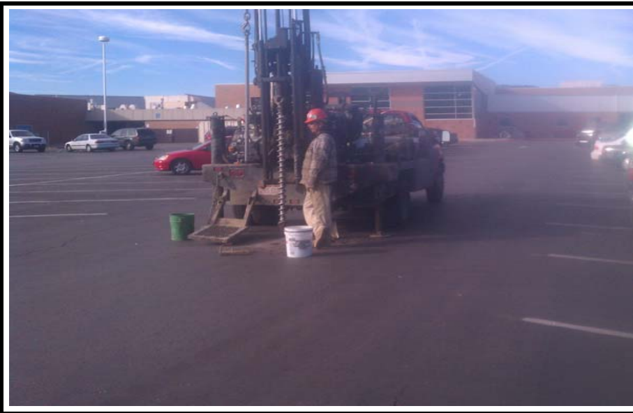
PHOTO NO. 3: View of pavement in general vicinity of Boring No. B-8. Pavement distress generally consisting of longitudinal and transverse cracking.
